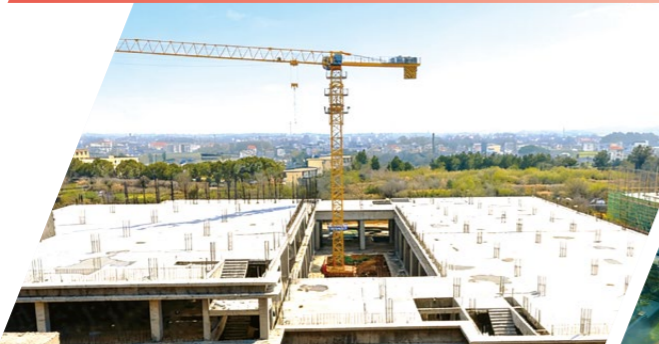
EPC General Contracting Project for the Liujia Mountain Smart Science and Innovation Park in Duchang County
