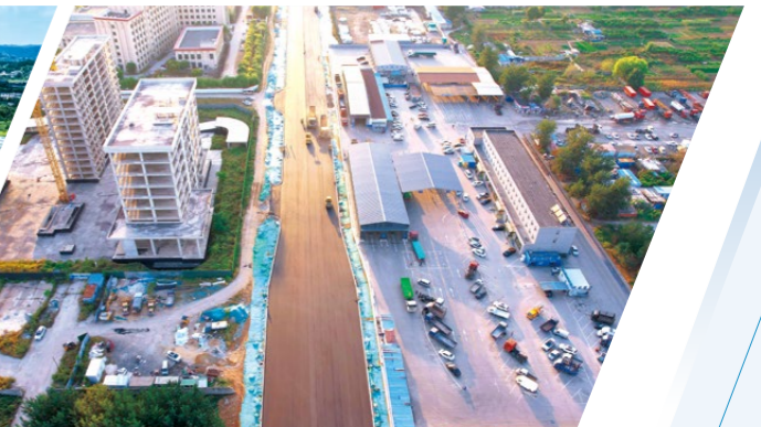
Infrastructure and Supporting Facilities Construction Project (Phase II) in Western Economic Development Zone in Lubei District, Tangshan City
