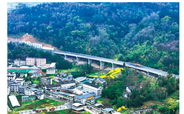
Pavement completed on Longxi Bridge under the Rural Revitalization Road Project in Nanshan Village, Emeishan, Sichuan Province
