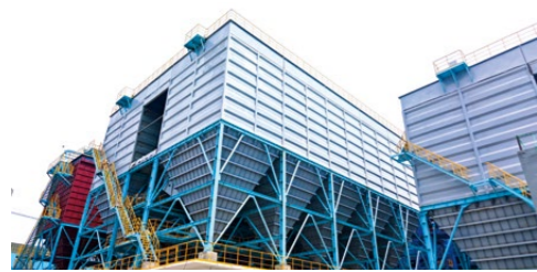
Zero-Carbon Environmental Protection BOO Project
