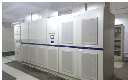
Converter Secondary Dust Removal System
